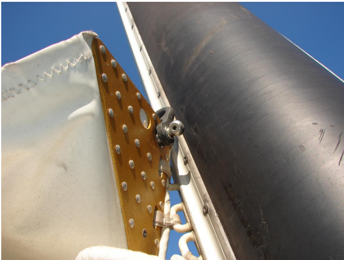
Photo 1. Minor cracking on a Freedom 39 mast, spacing about an inch apart.
